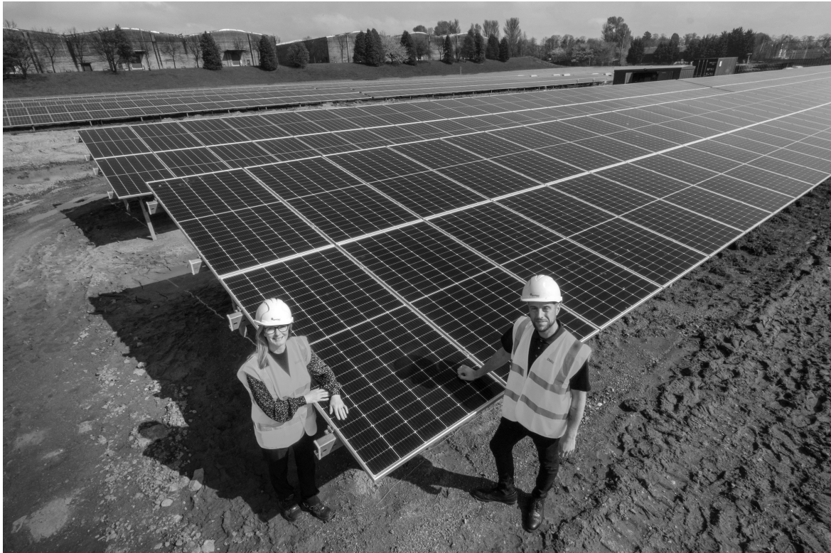
8,000 panel solar array at Diageo in Leven, Fife
